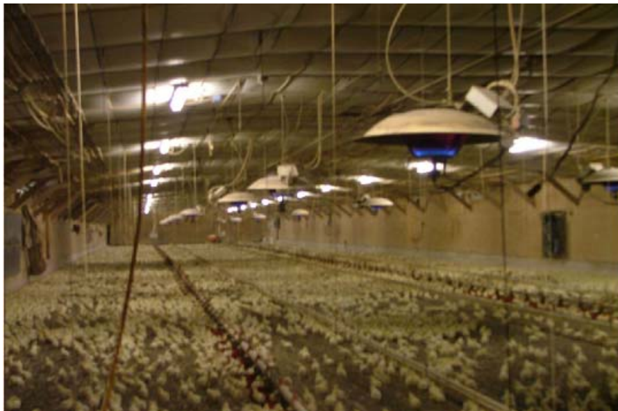
Figure 7. Chicken house with space heaters at the Frye Poultry Farm. 103
