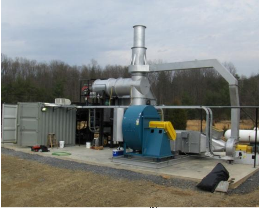
Figure 8. Gasifier at the Frye Poultry Farm. 104
