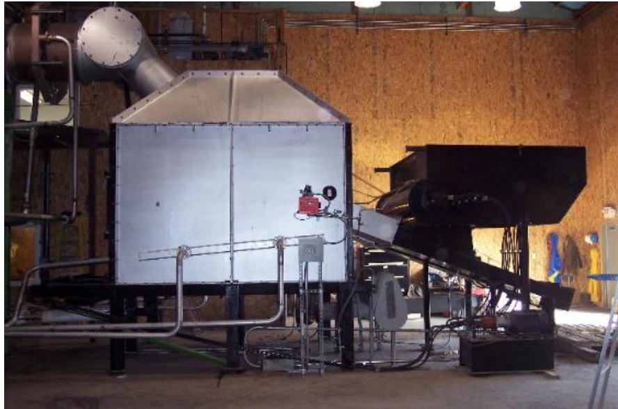
Figure 5. Primary gasifier unit. 97
