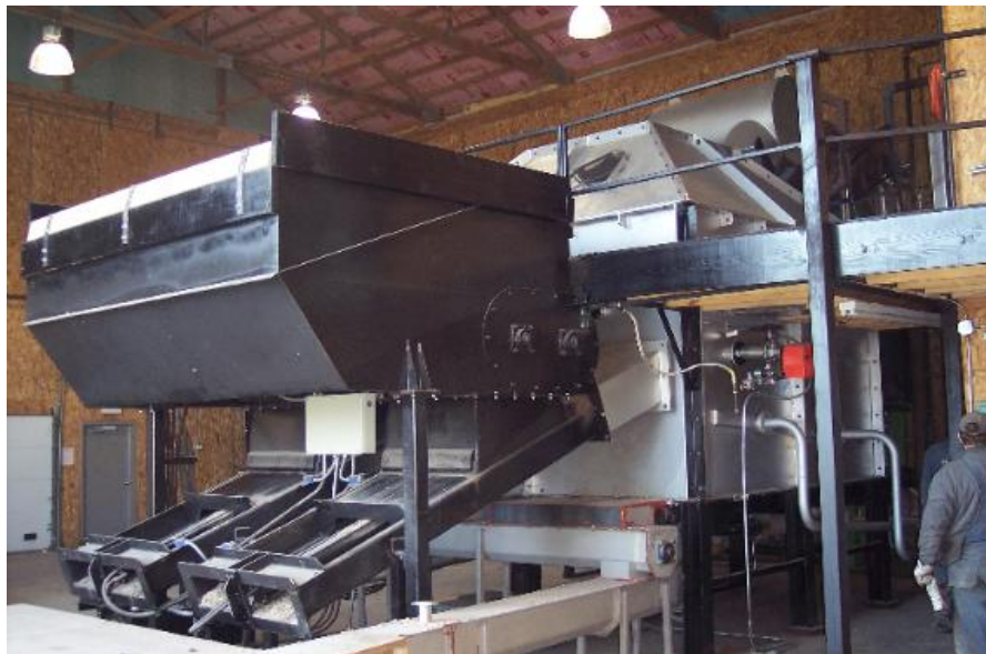
Figure 6. Front of gasifier and feed hopper. 98
