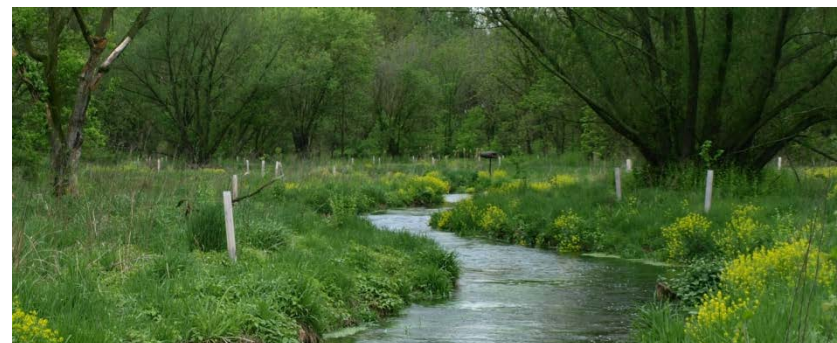
Floodplain restoration constructed in 2005 includes 1,800 linear feet of stream, wetland creation, riparian planting, and significant flood and deposition storage.
