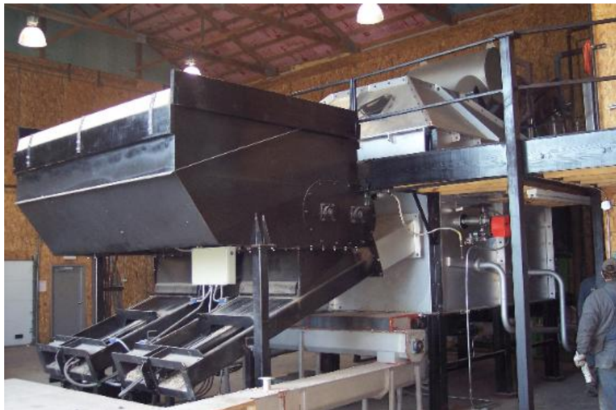
Figure 6. Front of gasifier and feed hopper. 98
