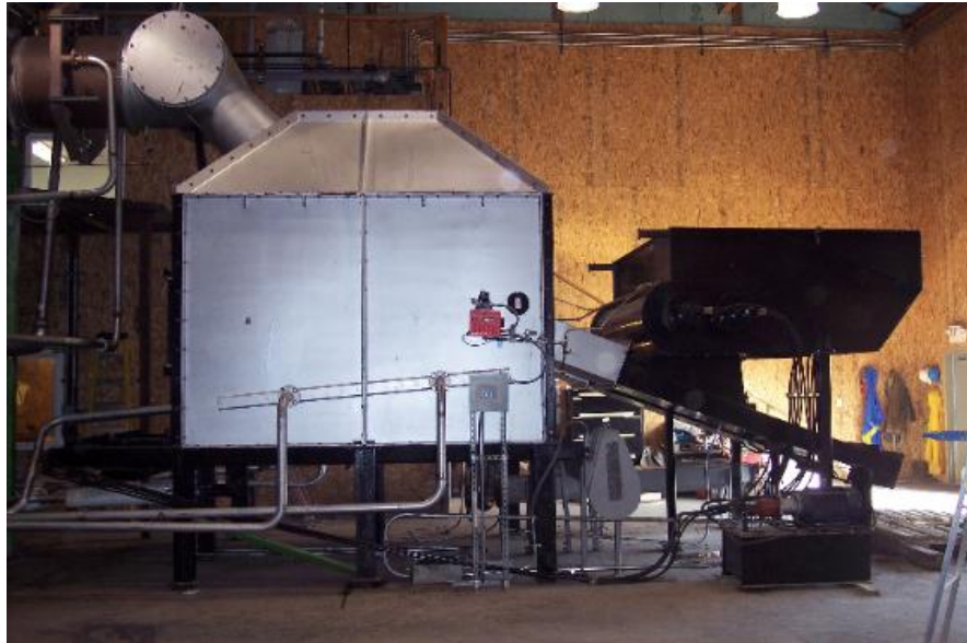
Figure 5. Primary gasifier unit. 97
