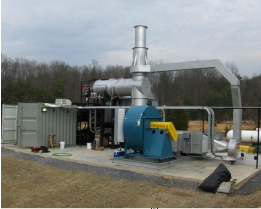
Figure 8. Gasifier at the Frye Poultry Farm. 104
