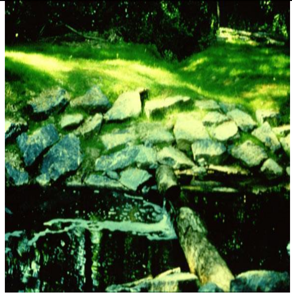
(b) Upstream Passage of Fish and other Aquatic Life can be Impeded by Poorly Designed In-stream Structures that Create Vertical Drops
