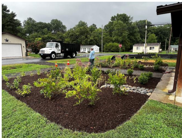
Images: Jonestown Community Stormwater and Resilience Project Source: Amanda H. Pollack, P.E., Center for Watershed Protection
