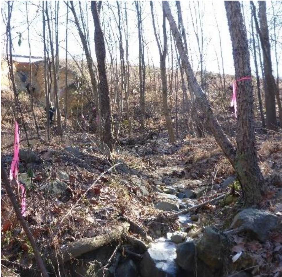
PRE - CONSTRUCTION: ERODED ROADWAY EMBANKMENT, SPRING 2016
