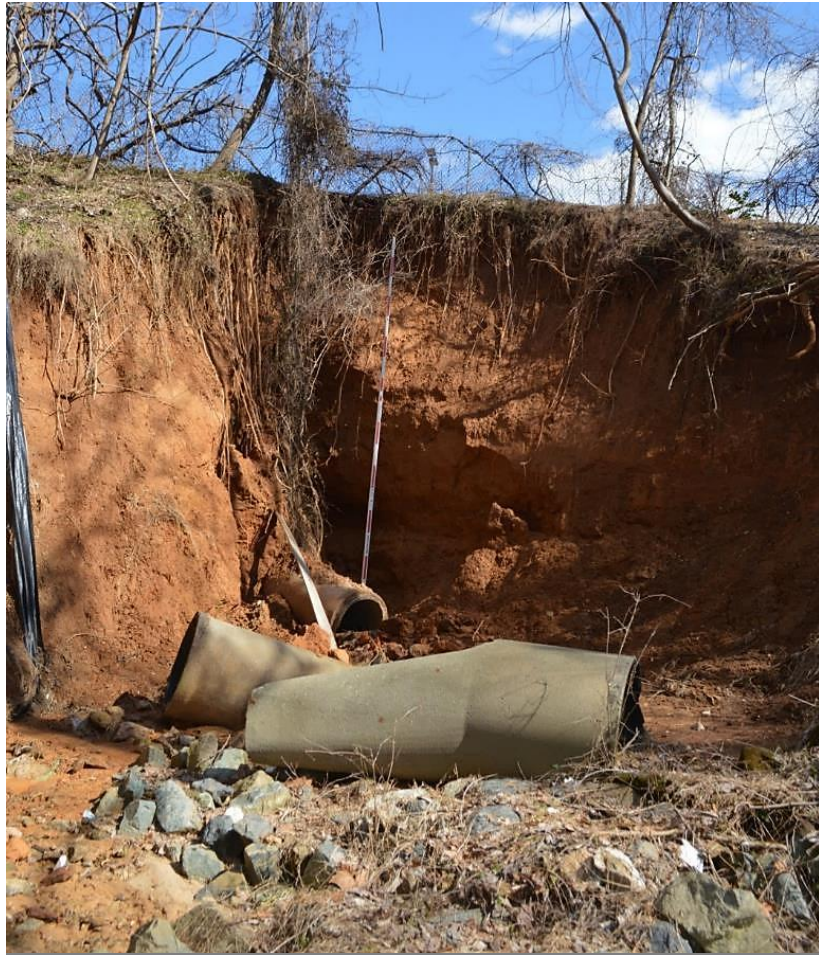
PRE - CONSTRUCTION: EXISTING EXTREMELY INCISED VERTICAL WALLS AND FAILED OUTFALL STRUCTURE , 2/29/2016
