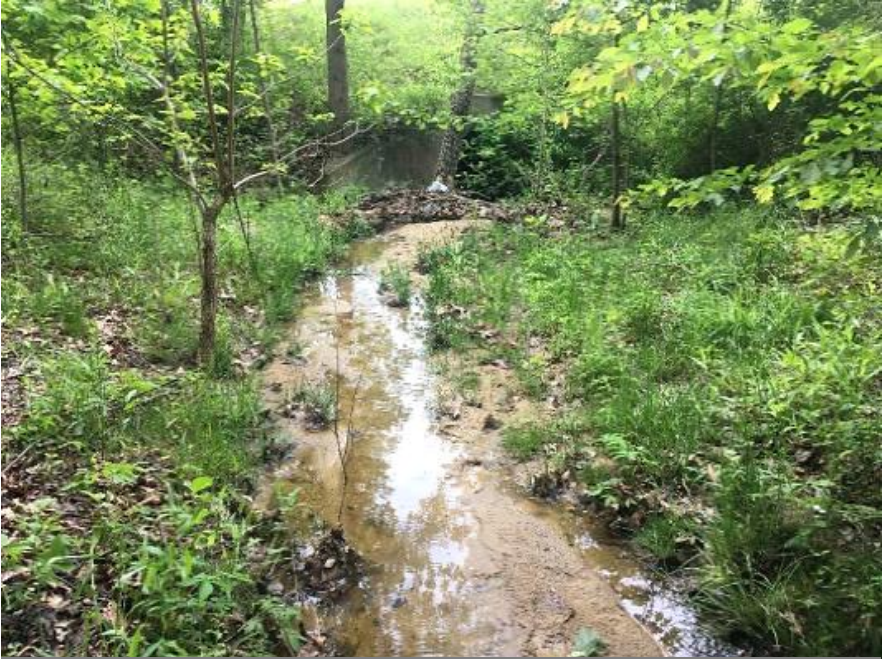
PRE- CONSTRUCTION: SAND GRAVEL DEPOSITION AT DOWNSTREAM CULVERT 5/18/2016
