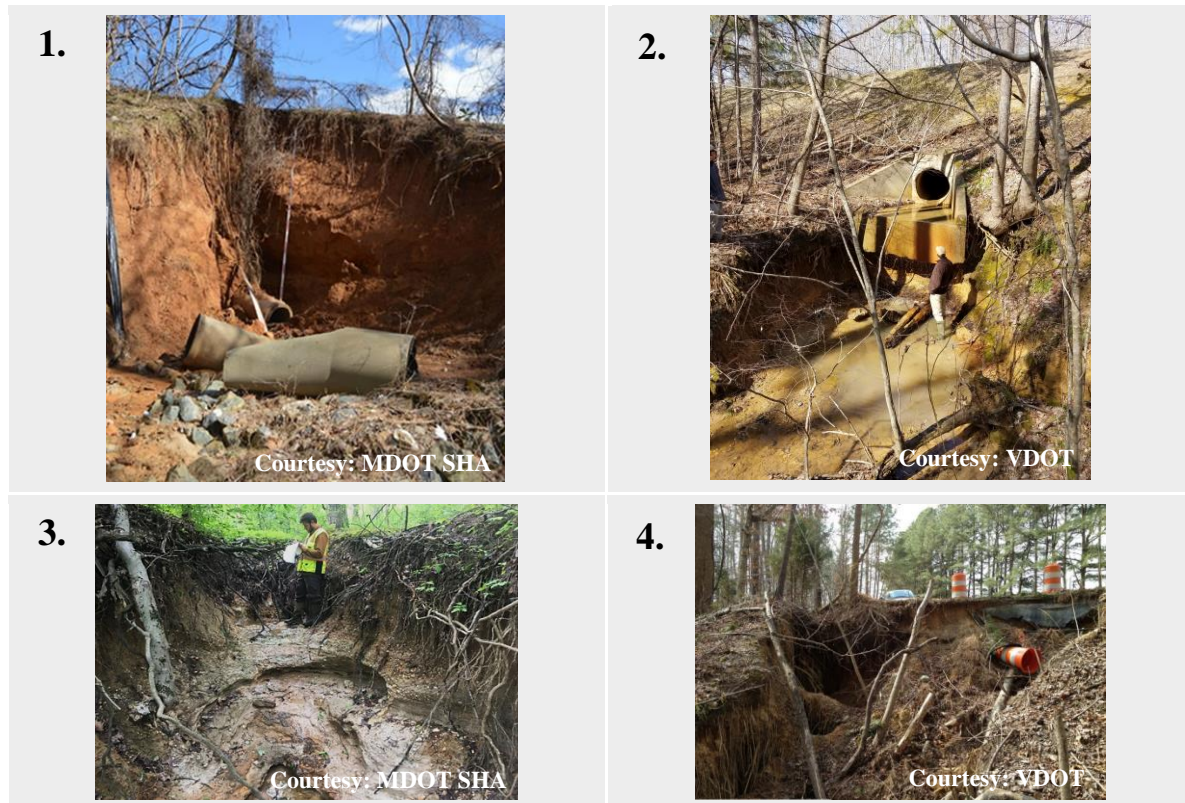
Figure 2. Examples of Severe Outfall Erosion in the Headwater Transition Zone
