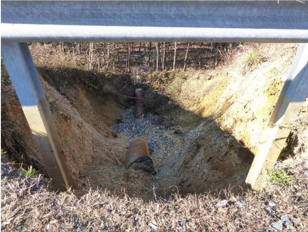
PRE - CONSTRUCTION: FAILED PIPE AND ERODED ROADWAY EMBANKMENT , SPRING 2016
