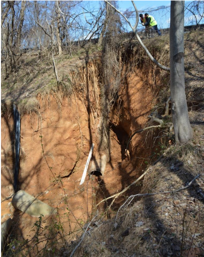
PRE – CONSTRUCTION: EXISTING EXTREMELY INCISED VERTICAL WALLS AND FAILED OUTFALL STRUCTURE, 2/29/2016
