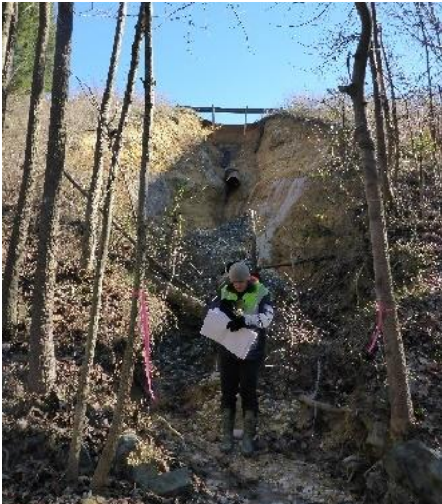
PRE – CONSTRUCTION: ERODED ROADWAY EMBANKMENT , SPRING 2016
